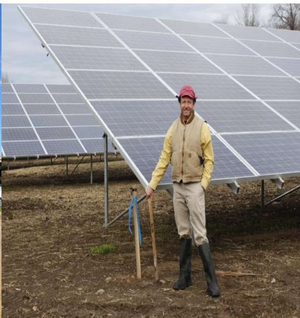
Ground Mounted 129 kW solar array at Freund's Farm, E. Canaan, CT. First Farm in CT to Virtual Net Meter. Additionally the farm has installed a 223 kW roof mounted array on their new robotic milking barn.
