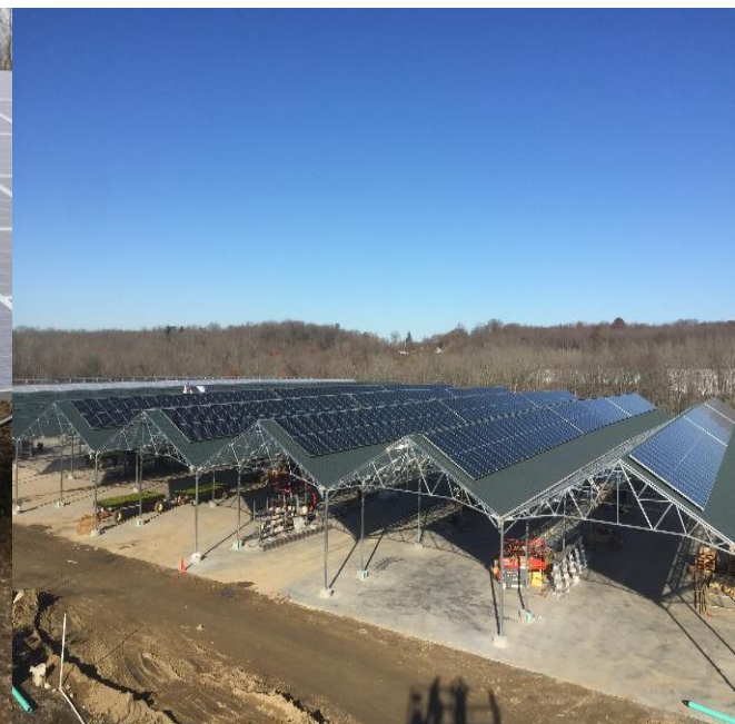
Prides Corner Farm in Lebanon, CT installing 240 kW solar system on a newly constructed greenhouse structure.
